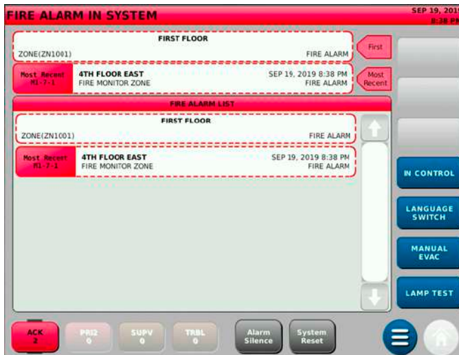
Figure 7: First and Most Recent Alarm Display
